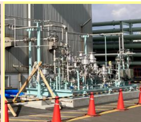
SVT (Supply Valve Train)
